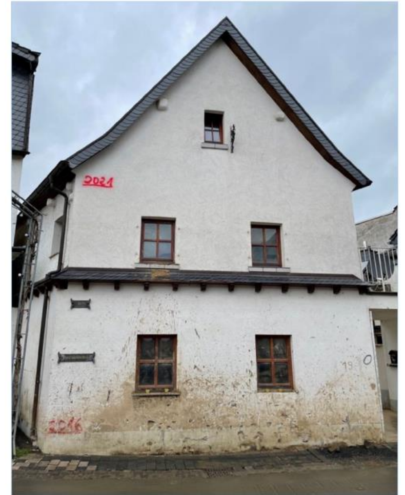
Flood markers at a central building in Dernau indicating the flood levels of 2016, 1910, 1804 and 2021 (bottom to top). Michael Szönyi, 5.4.2022.
